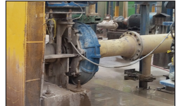
Pump operating leak free for over 30 days, saving the customer thousands of dollars.
