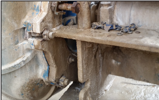
Pump leaked excessively.
